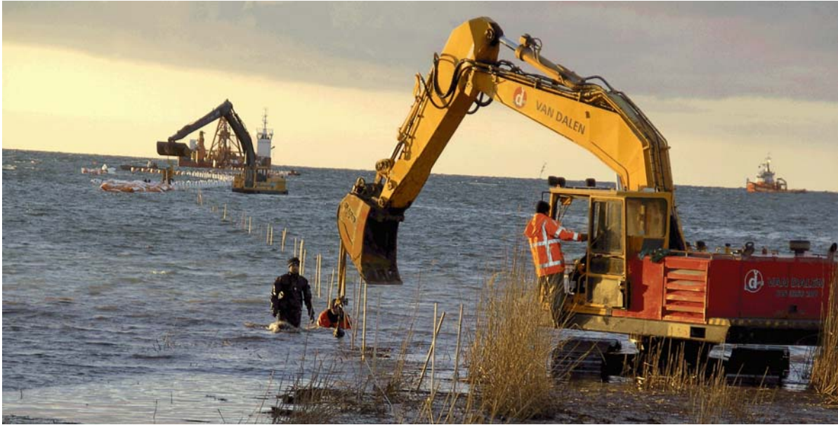
Figure 14. The cable pull-in at the shoreline made by the excavator and a pull-in winch.
