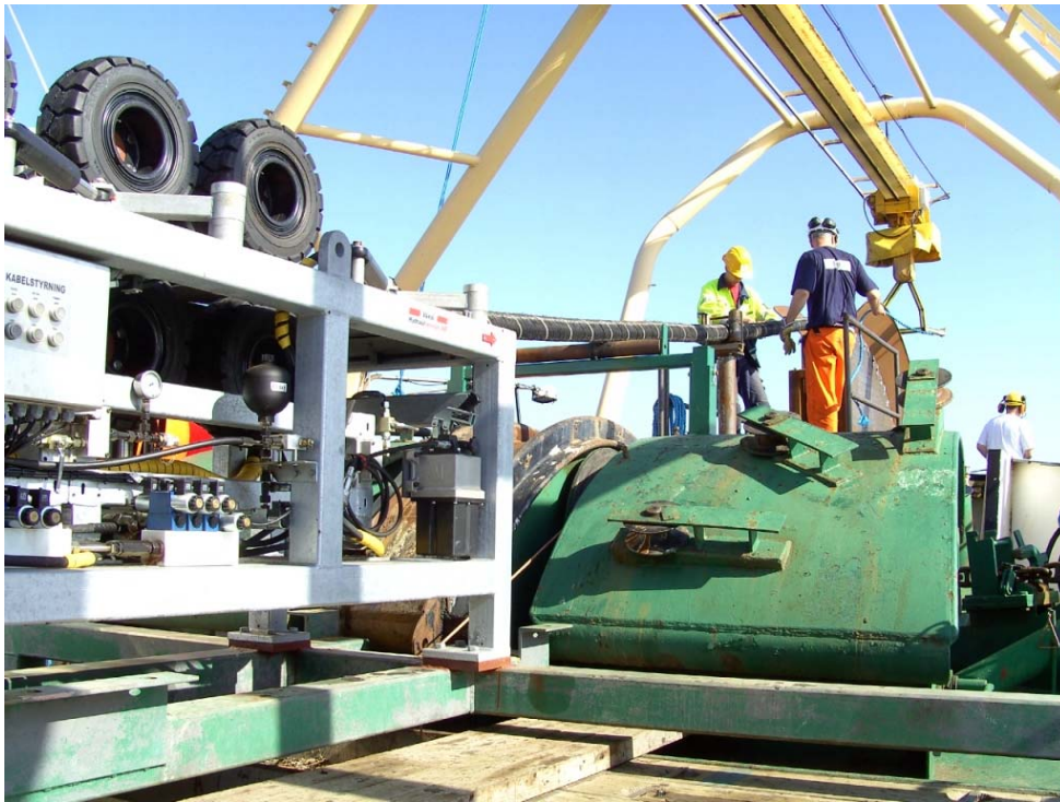
Figure 18. The linear cable engine transports the cable forward to the bow wheel.
