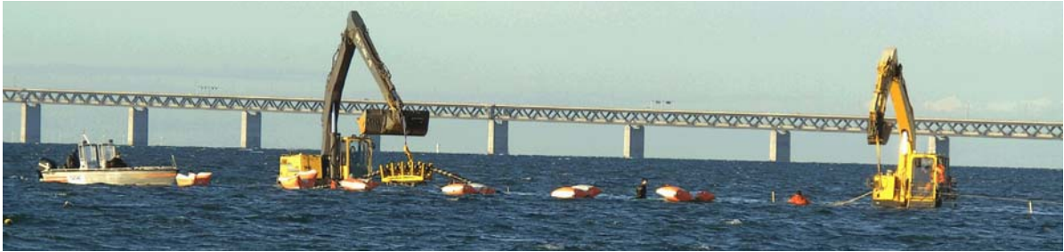
Figure 13. The cable pull-in made by the excavators and a pull-in winch. A bigger workboat and two divers were also used.
