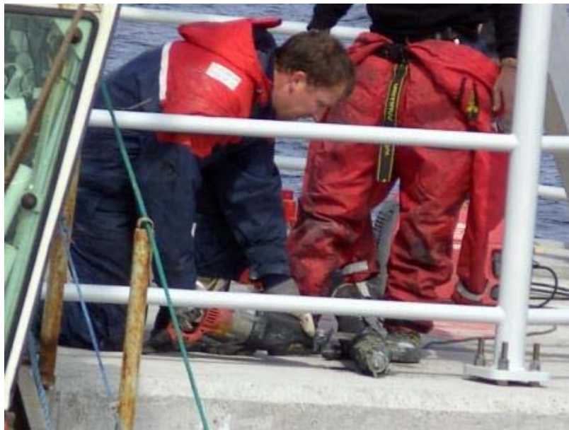
Figure 27. A tiger saw was used to cut the excess length of cable
