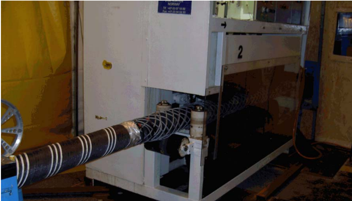
Figure 8. In a tent on the quay a second pulling device was placed. In the tent the cable was marked at exact lengths.
