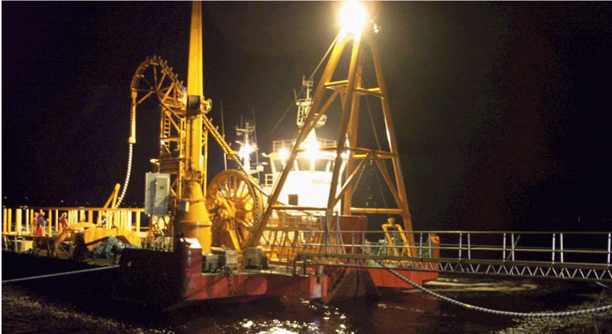
Figure 9. To the right of the picture is the slack from the quay. On the barge are the pulling devices, the capstan and the vespa on the “gooseneck”.
