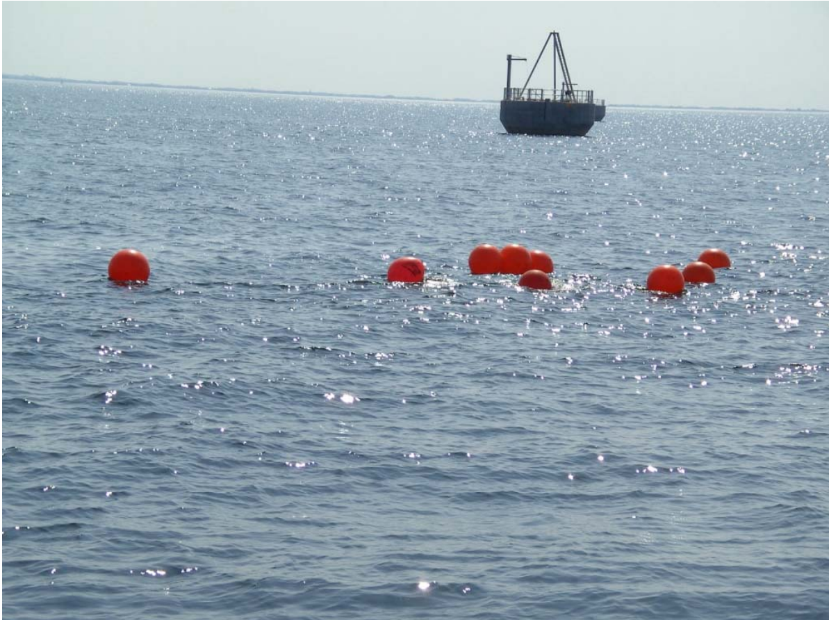
Figure 22. The water current affected position of the cable and the floaters during the pull-in.
