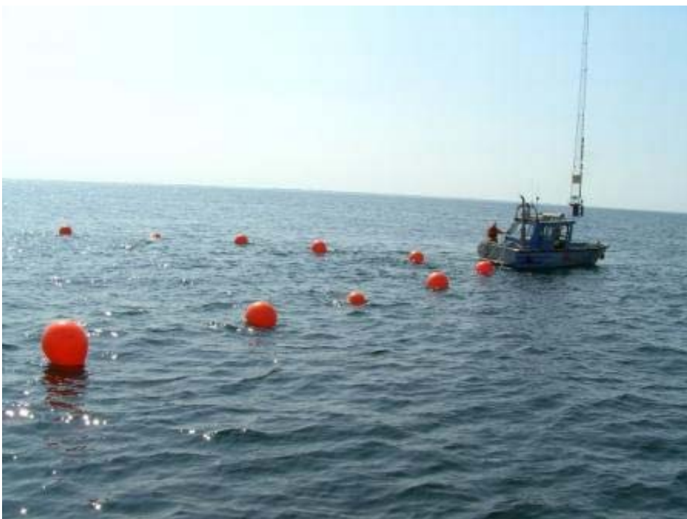
Figure 25. A workboat pulled the cable to minimise the risk for a kink
