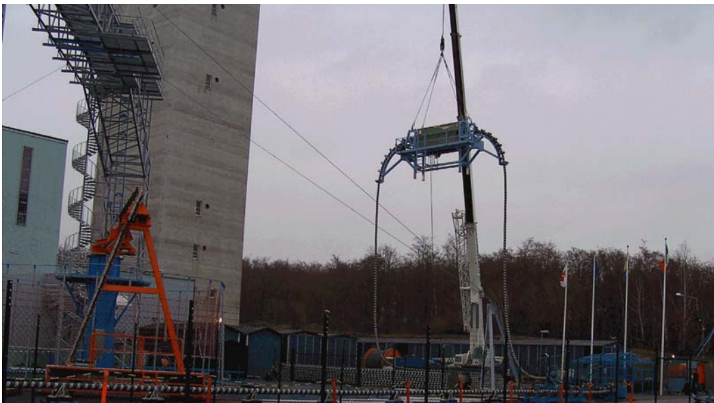
Figure 7. The cable engine hanging in the crane pulled the coiled export cable from the storage space. As can be seen above, the cable is transported 400 metres on conveyor idlers.
